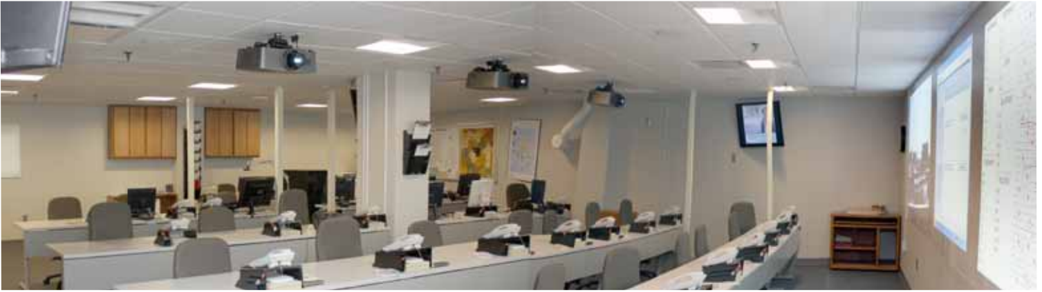
Stations for 28 staff were included in the new Lancaster County Emergency Operations Center.
