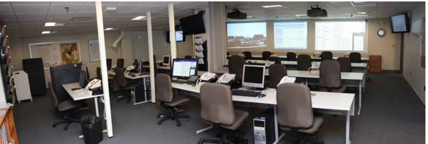
A view from the back of Lancaster County's new Emergency Operation Center in Lincoln.
