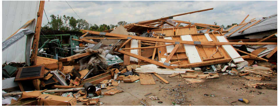
Sarpy County damage included destruction at Papillion's Waste Water Treatment Plant.
