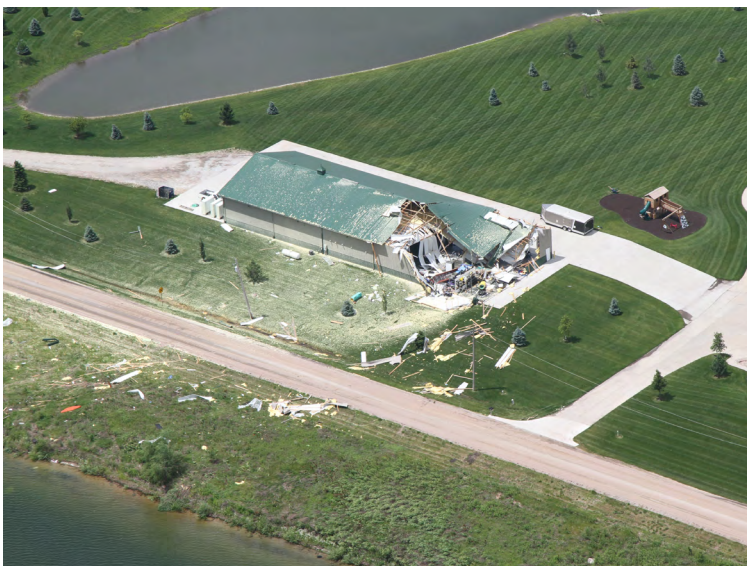
The June tornado caused roof damage in Cass County.
