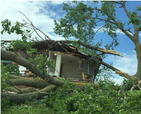
A tornado damaged Bellevue's Rising View neighborhood during June storms.
